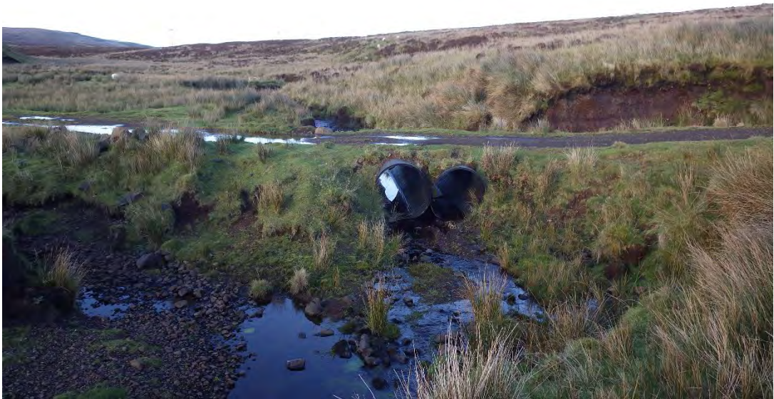
Photograph 9.4.2 View of original river channel and current twin pipe culvert crossing. View N from NGR NG 3075 4694.
